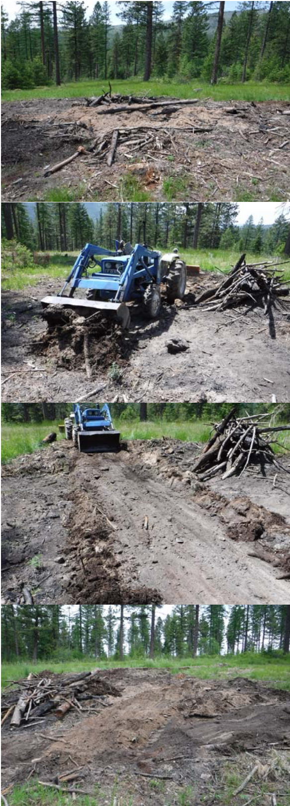
Fig 3. Rehabilitating a burn pile with a small tractor can take less than 1/2 hour.
